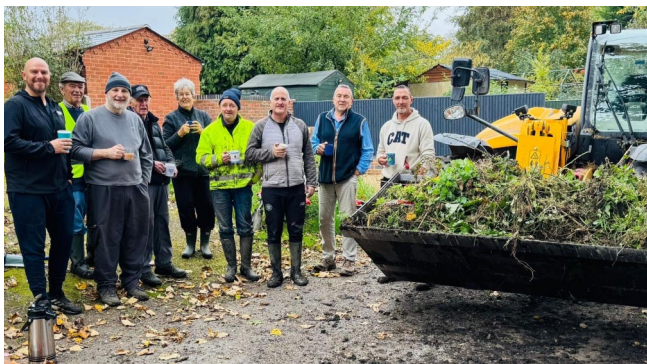
The drain gang take their customary coffee and cake break after (a hard morning) clearing the stream along Moor Lane
